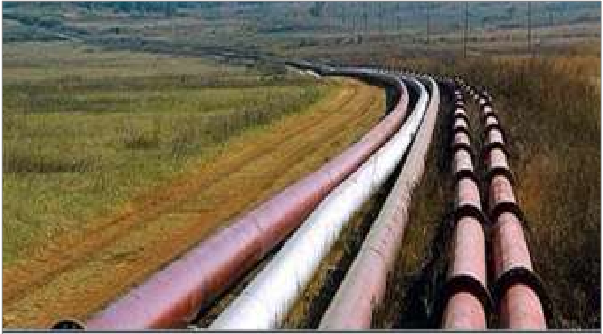
Figure 78: Above Ground Pipeline System
