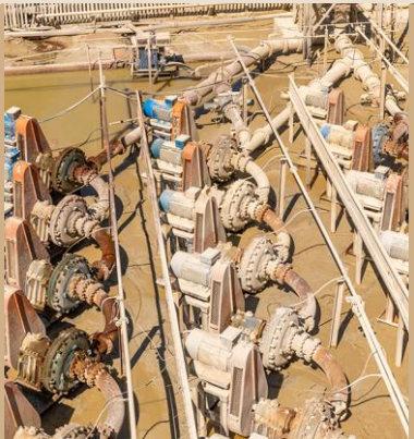
Slurry mix pumped to reduction works through network of pipelines
