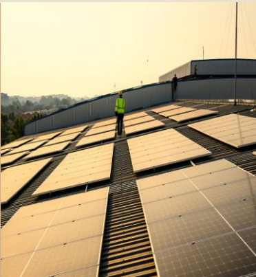
Energy generation - PV facility
